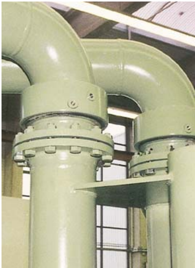
STENFLEX Swivel Joints type DG-02S installed at loading arms
